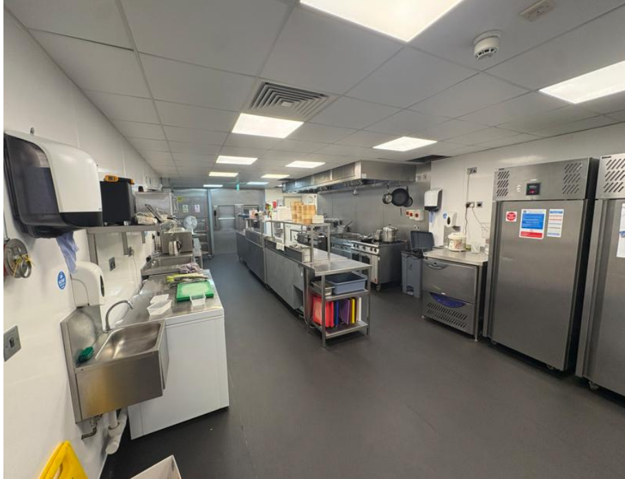
First Floor Main Kitchen Area
